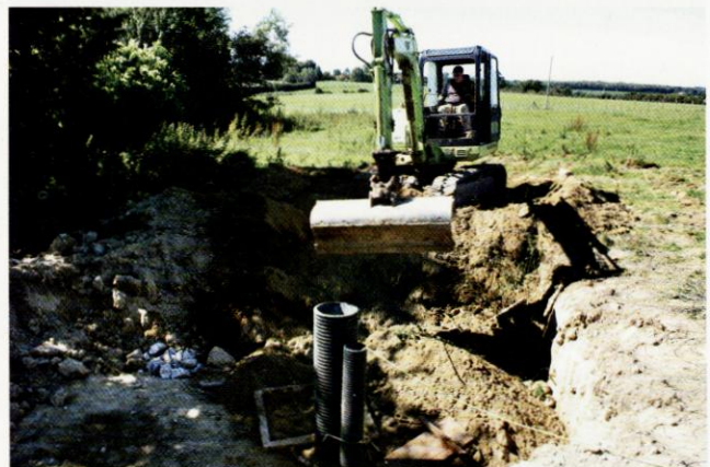
Good as new – you'd hardly know we'd been here after six months. The next job is to build a surface utilities point and a short 'chimney' to help draw air through the bunker.
